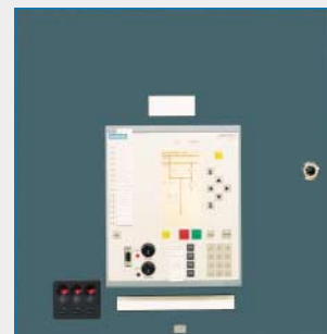
Siemens type Siprotec protection relay.
