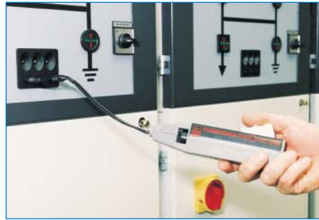
Testing the LED voltage indication.
